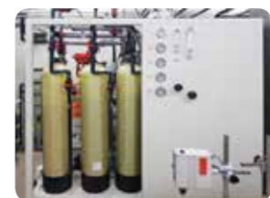
Pressure vessel polisher for RO unit
